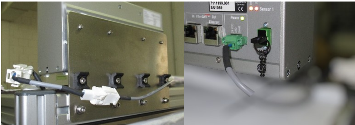
Figure 4: Left: Y-cable connected to 24 supply and to the fan, right: Connection to controller.
