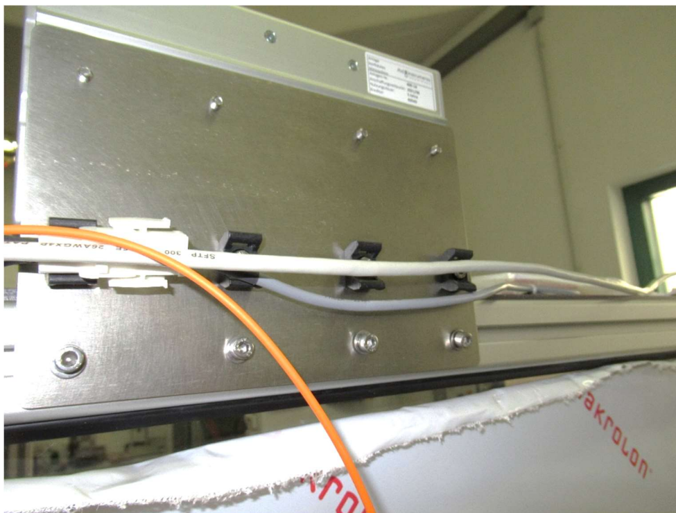
Figure 7: Fixing points for all cables at the backside of the sensor support plate.
